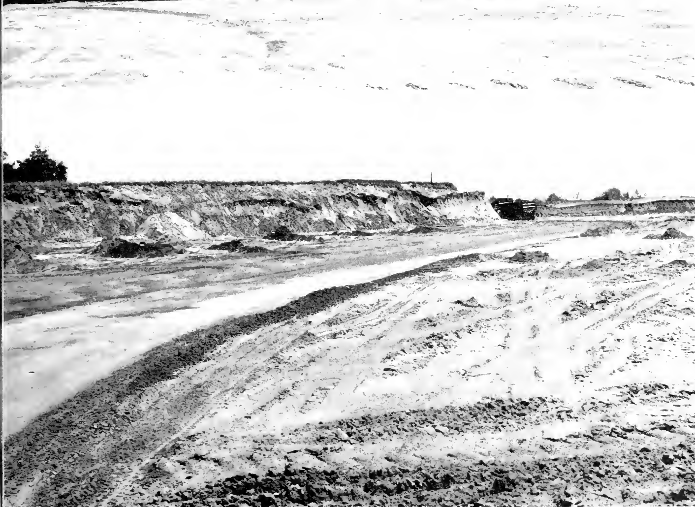
UPPER—Loading with a crawler-type belt loader pulled by a tractor. LOWER—Area of maximum cut showing high, previously unirrigable land being improved to an irrigable graded plane.
